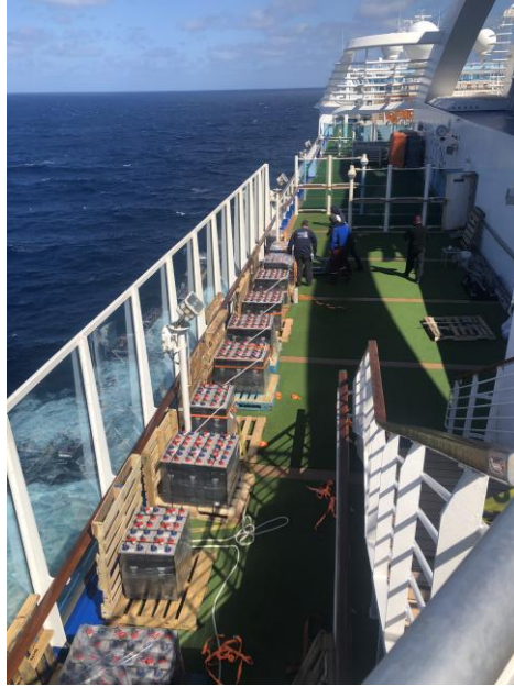
Figure 2: Batteries staged for replacement on Ruby Princess (2024 Photo by Norbert Doerry)
